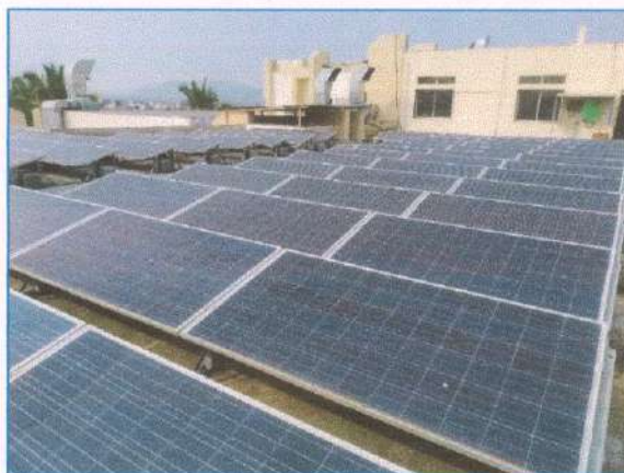
Photographs 8 : Solar System Installed at Institute
