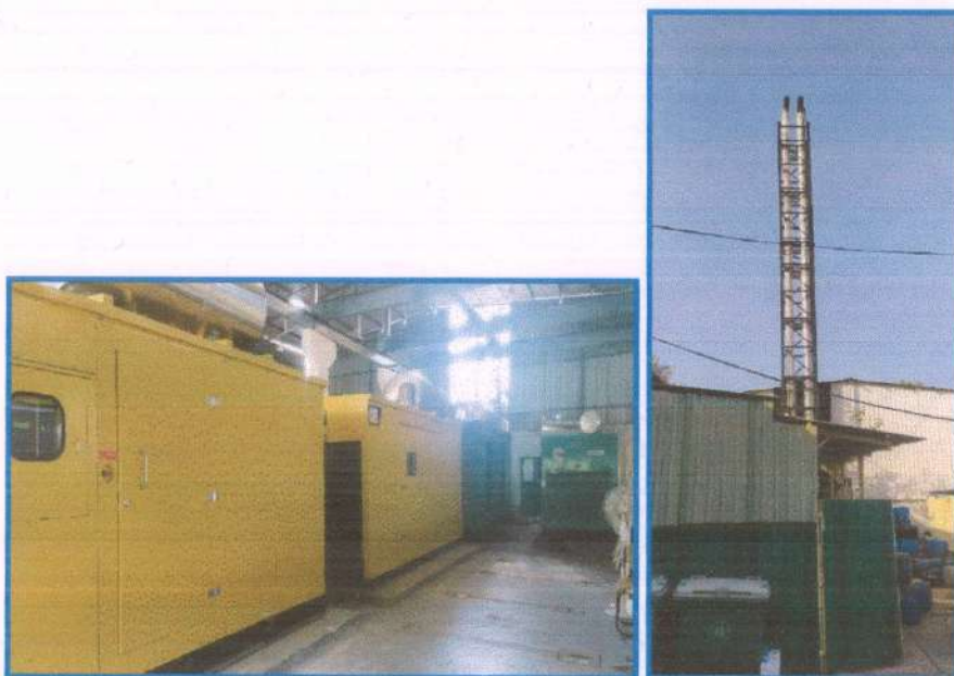
Photographs 4 : DG Set with adequate Stack Height as per Consent
